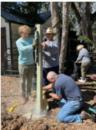
Garrett Nielsen (L) working hard with Jenneke Visser and Clay Smilie to erect posts for the new fence.
